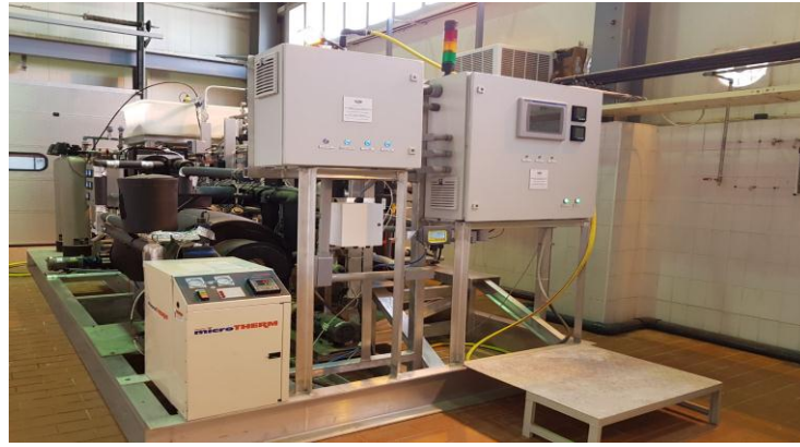
Plate 1. Investigated pilot test unit at Desalination Research Plant (DRP).
